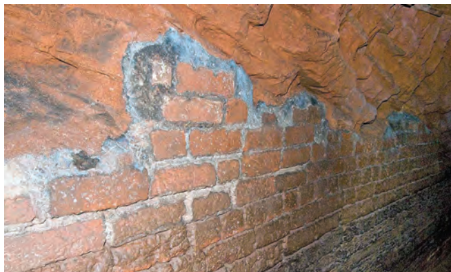
Some sections of the tunnel wall have been reinforced with brick. Was this due to boat damage or just a soft patch of sandstone?
